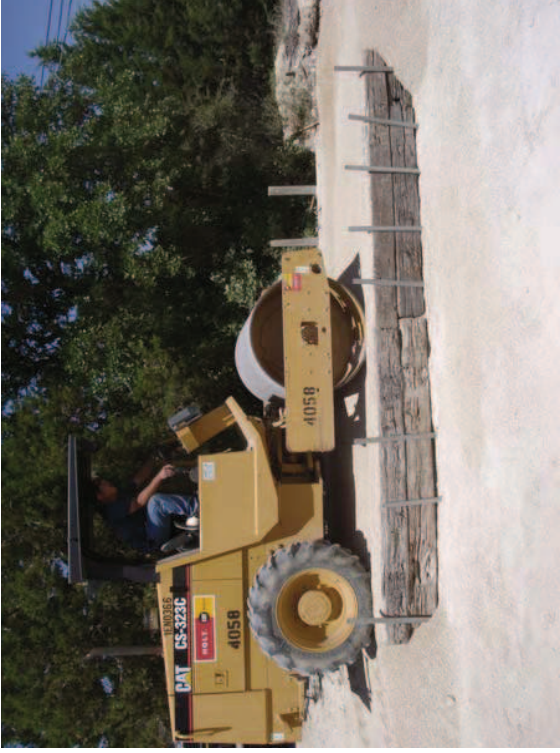
COVER SOIL/AGGREGATE IS UNIFORMLY SPREAD AND COMPACTED USING FIELD-SCALE EQUIPMENT AND PROCEDURES
